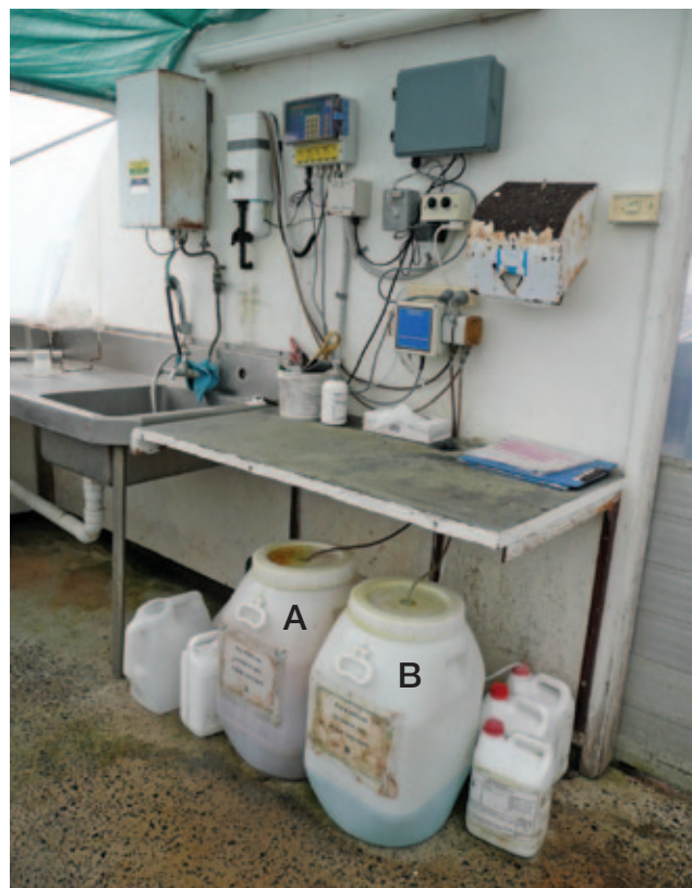
Tanks A and B containing concentrated stock solutions are shown here with a nutrient controller mounted on the wall to automatically dispense the stocks into fresh water to make the working nutrient solution.
