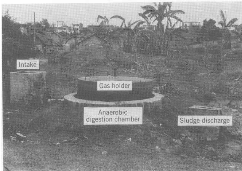
FIGURE 15.13 Biogas generator with intake hopper (at left), floating metal gas holder and anaerobic digestion chamber in the center, and sludge discharge at the right.
